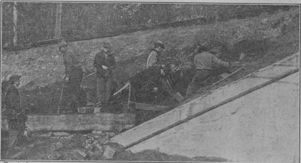
Track Gang "Cribbing" the Roadbed at Summit, under the Direction of Mr. Nees, Familiarly Known as Carl (Facing the Camera). There Isn't Much Around a Small Railroad That Carl Can't Do. Cribbing Keeps a Roadbed from Sliding Down an Embankment
