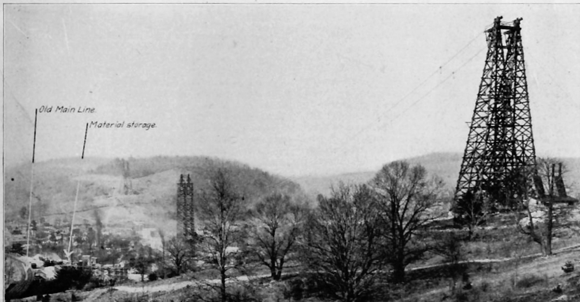
General View of Tunkhannock Viaduct Location, Showing End Tower and Operator's House of Material Cableway in Foreground
