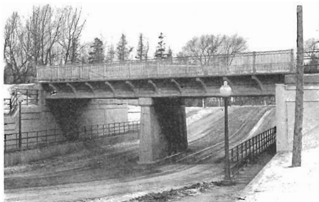
The Bridge Over La Canardiere Road, Which Has Precast Deck Slabs From 30 \frac{1}{2} Ft. to 37 \frac{1}{2} Ft. Long
